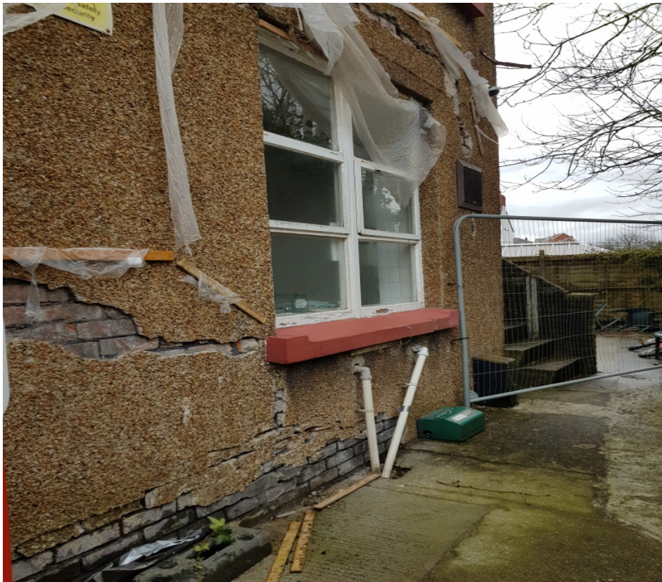
External Wall pending repair
