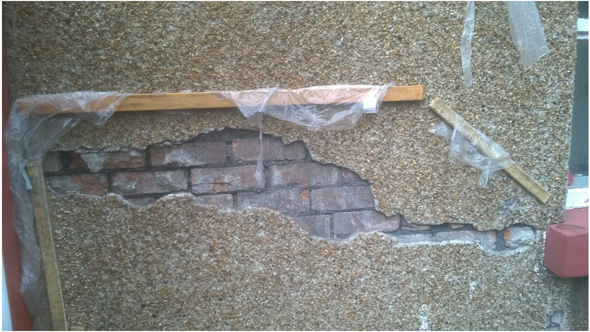
External Wall pending repair
