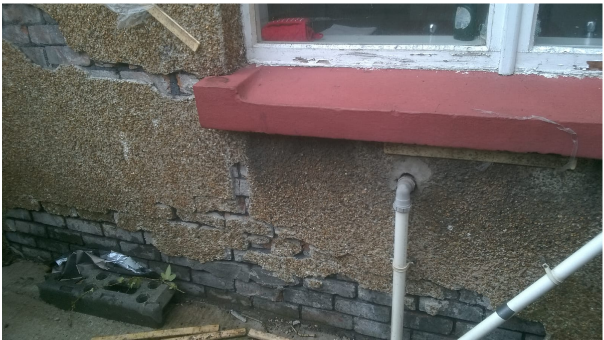
External Wall pending repair
